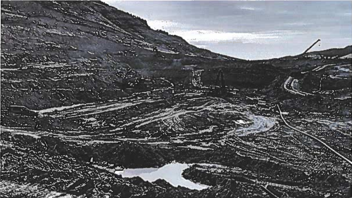
Excavation at the main dam has started to expose and clean the bedrock foundation.
