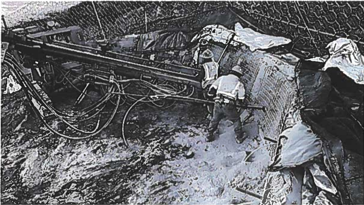
Construction has started at the downstream tunnel portal so that tunneling can begin at the start of the new year. Ultimately, the tunnel will be used to get water in and out of the dam.
