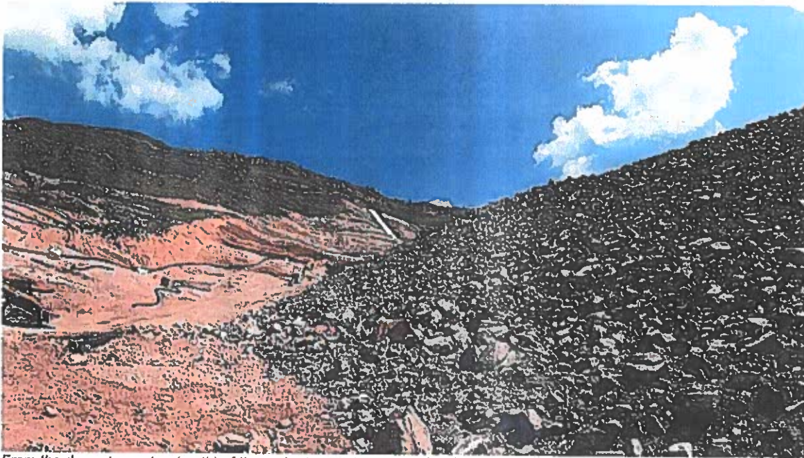
From the downstream toe (north) of the main dam embankment, looking west toward the right abutment.
