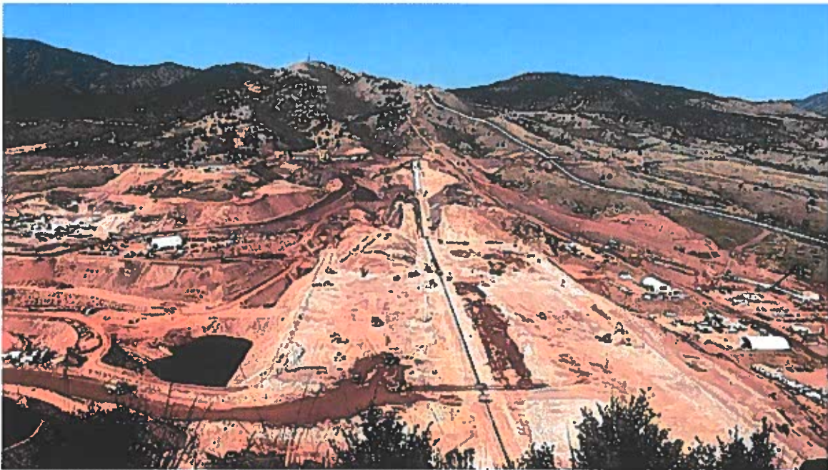
Construction on the Chimney Hollow Reservoir Project has reached the half way mark.
