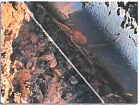
195' west of 19 where tar paper fell off in sheets.jjpg
