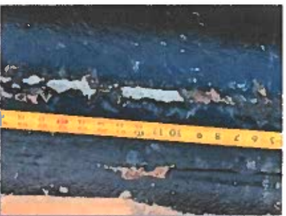
475-485 close up of damage to bare steel.jpg
