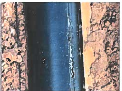
475-485 sewer tar damage into steel.jpg
