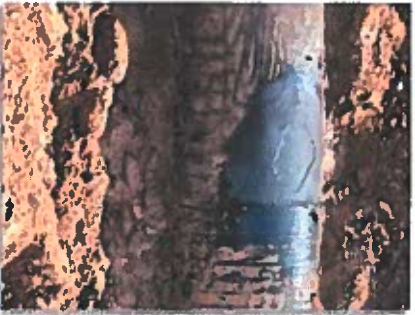
805 tar coating chipped away.jpg
