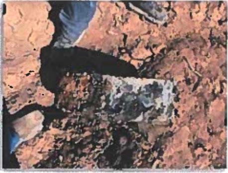
1260-1280 removed section of pipe found in trench by couplers.jpg
