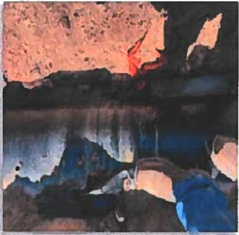
175-185 fiber along pipe with scrape in tar from top.jpg
