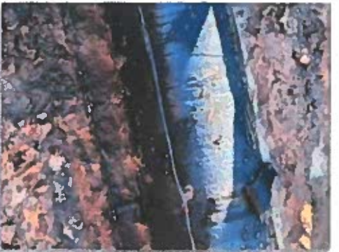
315 gouge deep into tar coating but no through to steel.jpg
