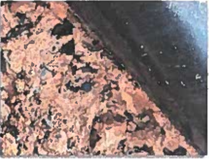
775 12' scrape on pipe no damage to steel tar only.jpg
