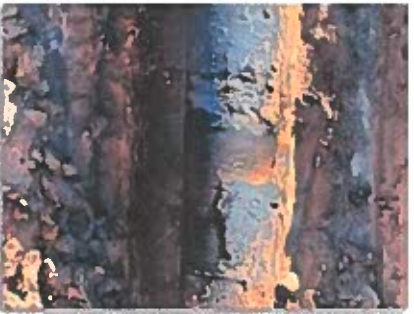
325 peeling tar coating.jpg
