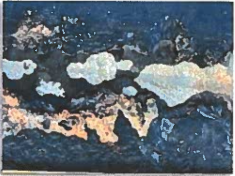
475-485 damage to steel.jpg
