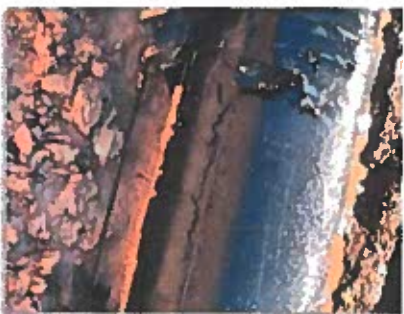
335 peeling tar below the score no bare steel.jpg
