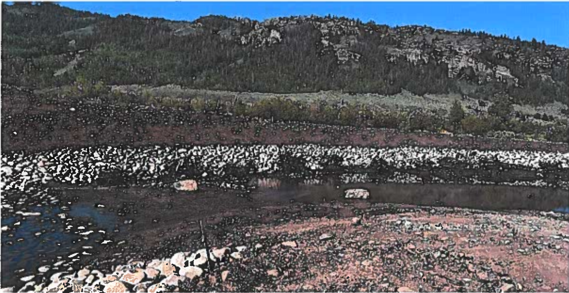
The Colorado River Connectivity Channel is on schedule to be substantially complete in 2024.
